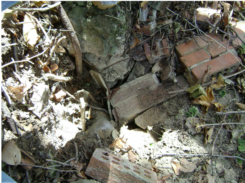
Junk in the Sinkhole
